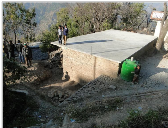
A north direction view of newly constructed house of Shri. Bhagwan Das, at the proposed site
